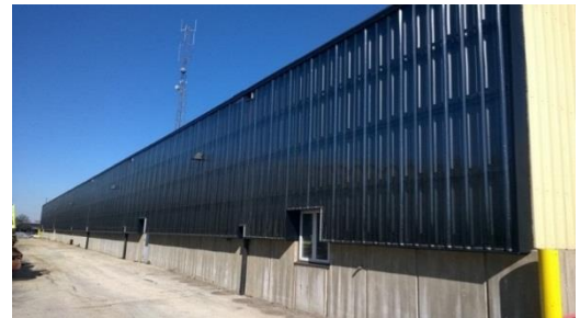
Schaumburg Department of Transportation and Highway Maintenance Facility Solar Thermal Wall
